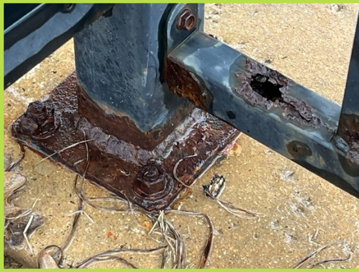
Base supports and anchor bolts are rusted through
