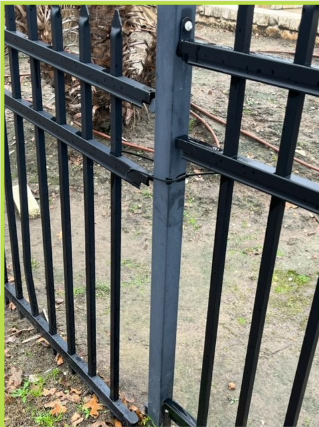
Fence is zipped tied together in several spots
